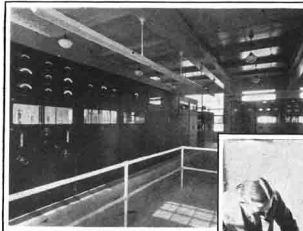
WHAT IS THIS—A POWER PLANT OR A RADIO STATION? —Just between ourselves, it is a radio station, and the most powerful broadcaster in the world at that. It is this view of the transmitting equipment that greet the visitor as he enters the front door of the main building. At the left is a long line of amplifier and oscillator panels. In the background is part of the power supply rectifier system which supplies high-voltage direct current to the plates of the tubes. Although now operating at fifty kilowatts, the equipment here pictured has sufficient reserve to enable WLW to broadcast with several times its present power.
